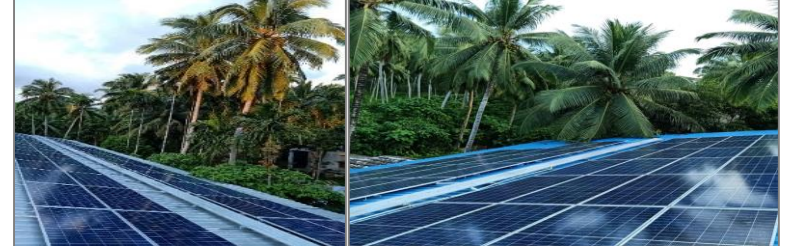
198 kW installation at Taj, Havelock Island, Andamans
