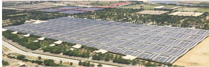
India's largest solar rooftop power plant: 16MWp at RSSB - EES, Amritsar
