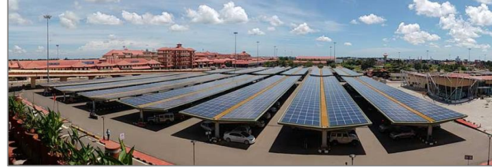
One of the Largest carport installations at an airport: 2.67 MW at Kochi Airport
