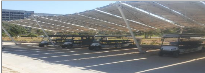
Solar EV Charging Station at Gujarat Sachivalaya, Gandhinagar
