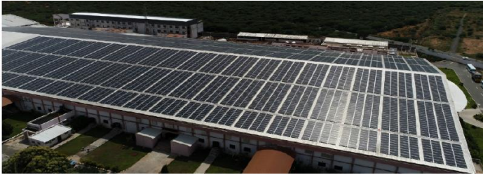
2.8MW Rooftop Solar Plant at Akshara Textiles, Tamil Nadu
